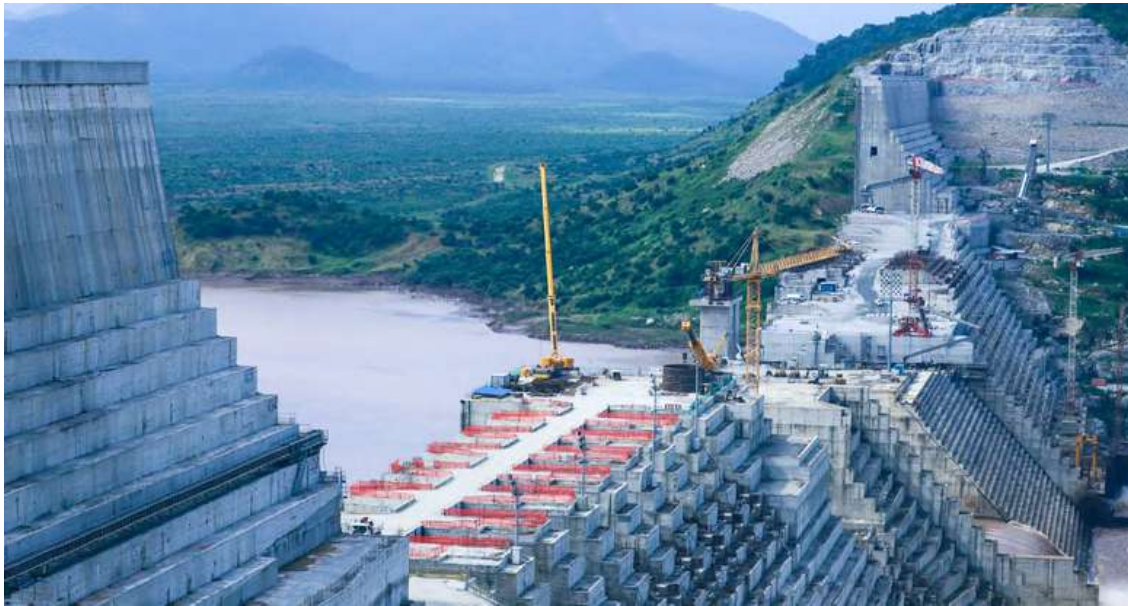
Ethiopia's Grand Renaissance Dam is seen as it undergoes construction work on the river Nile in Guba Woreda, Benishangul Gumuz Region, Ethiopia September 26, 2019. Picture taken September 26, 2019. Tiksa Negeri/Reuters.
